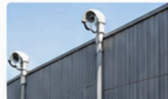
Perimeter & Security Integration with ONVIF surveillance systems
